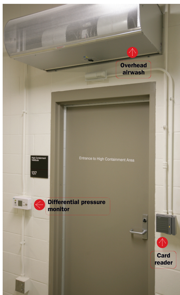
FIGURE 3. Containment Entry Vestibule with Overhead Airwash, Card Reader, and Differential Pressure Monitor*
