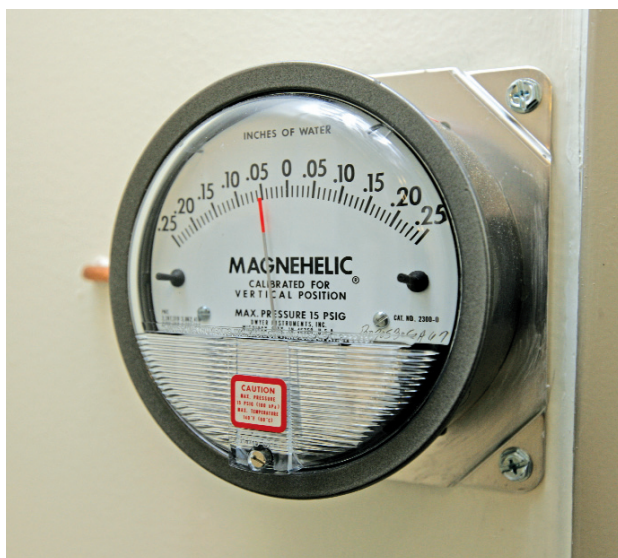
FIGURE 16. Magnehelic Gauge for Visual Confirmation of Pressurization
