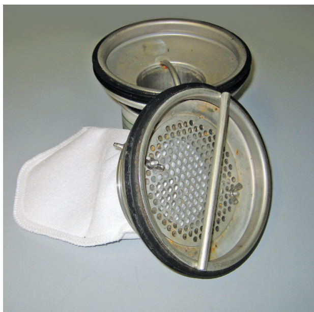
FIGURE 11. Filter Sock on Floor Drain*
