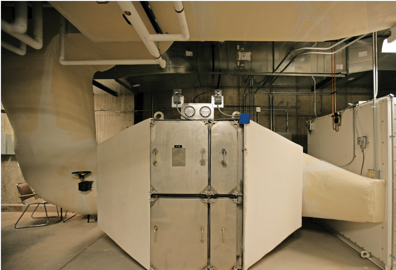
FIGURE 15. Bag-In, Bag-Out HEPA Filter System Attached to Air Handler*
