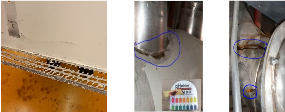
Figure 2: Corrosion of the mesh was observed after removal of the fume hood baffle during inspection. Inspection of the fume hood exhaust and ducts revealed heavy corrosion and leakage of corrosive materials from the ducts.
